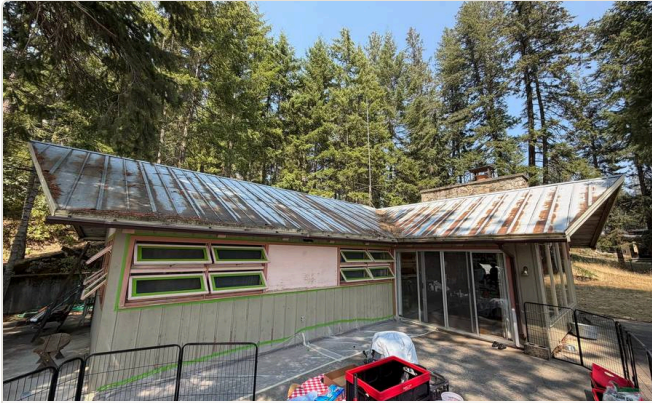
EXISTING METAL ROOF FROM GRADE: SURFACE CORROSION ACROSS THE PANEL FIELD
